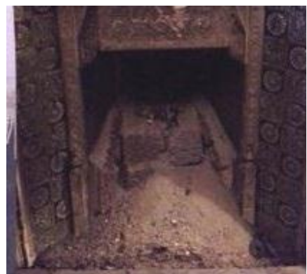
Carbon Monoxide risk from blocked flue found on testing of gas fire.
