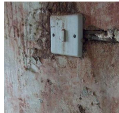
Health risk from cold, damp living conditions & electrical shock and fire risk from unsafe electricals.
