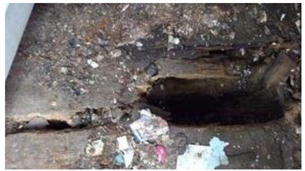
Trips and falls risk posed by holed and rotting floor directly in door entrance.
