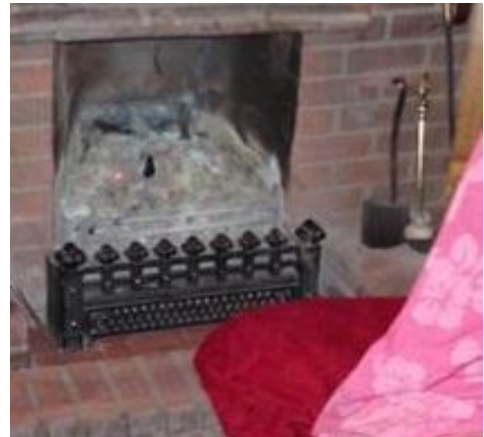
Excess cold risk of open fire being the only heating. Fire risk through absence of a fire guard.
